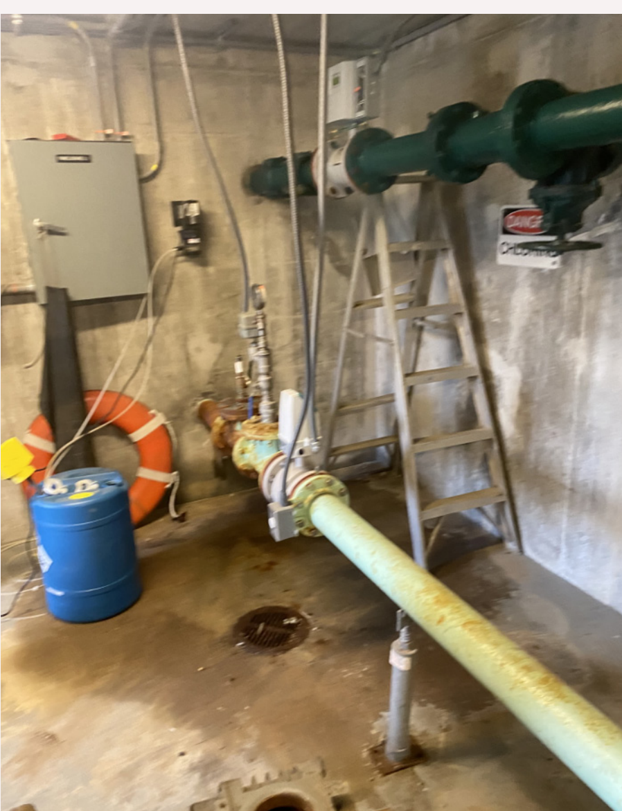
WWTP Chlorine Injection, Mechanical Piping and Flow Meter
