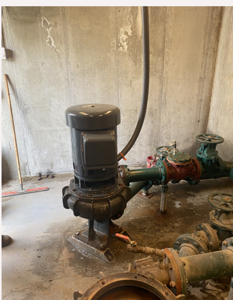
Lift Station Pump
