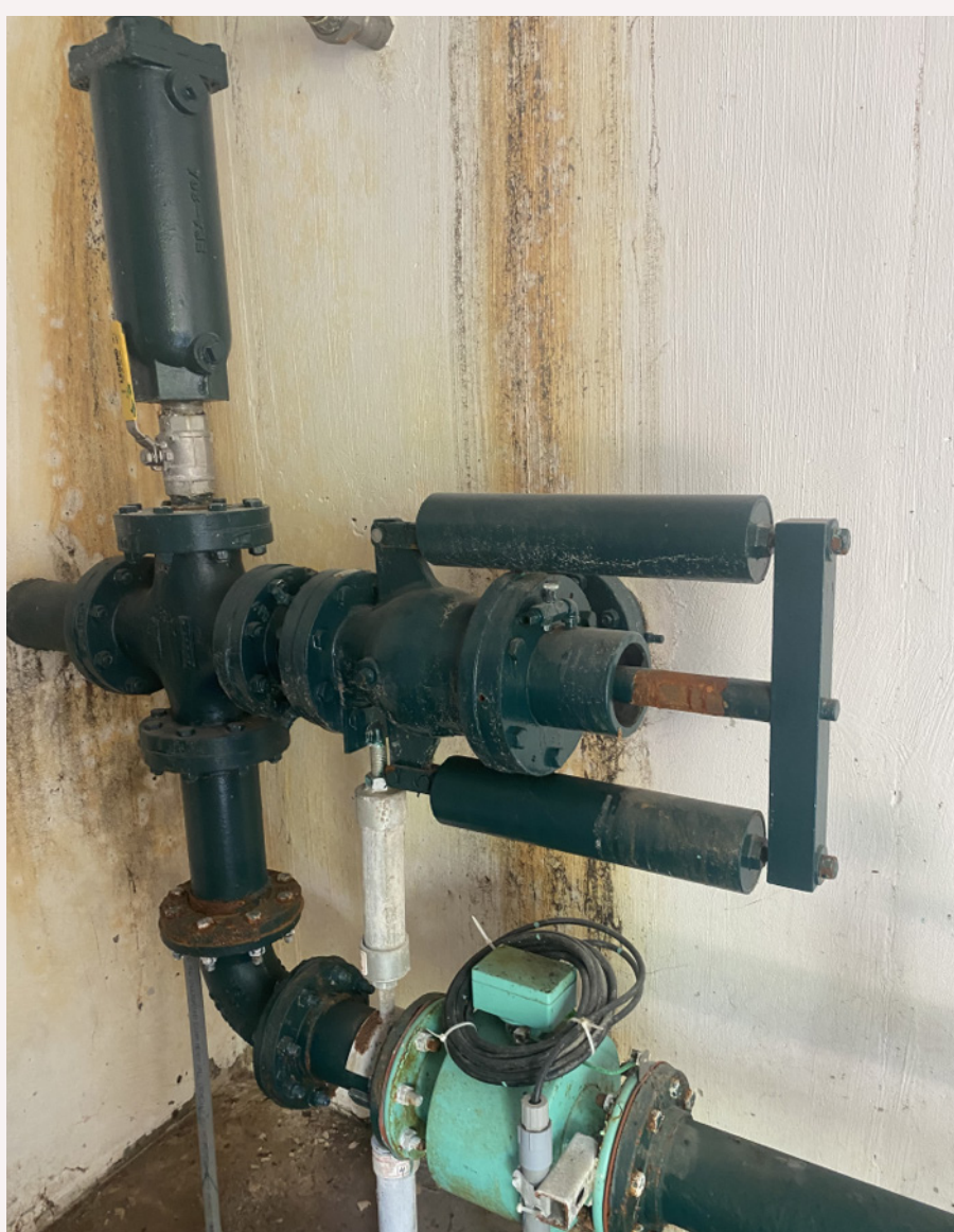
Lift Station Valving
