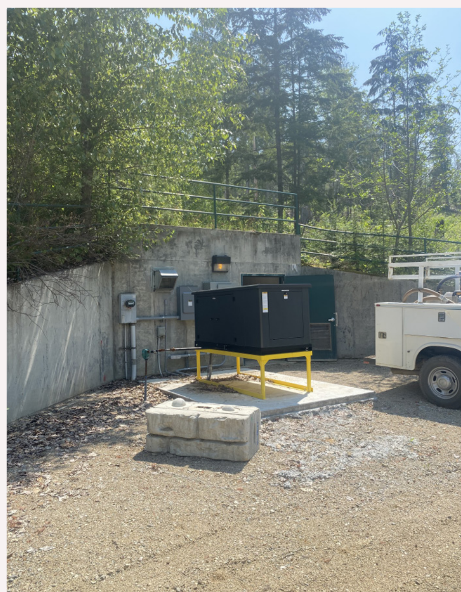
Lift Station Exterior with Backup Power
