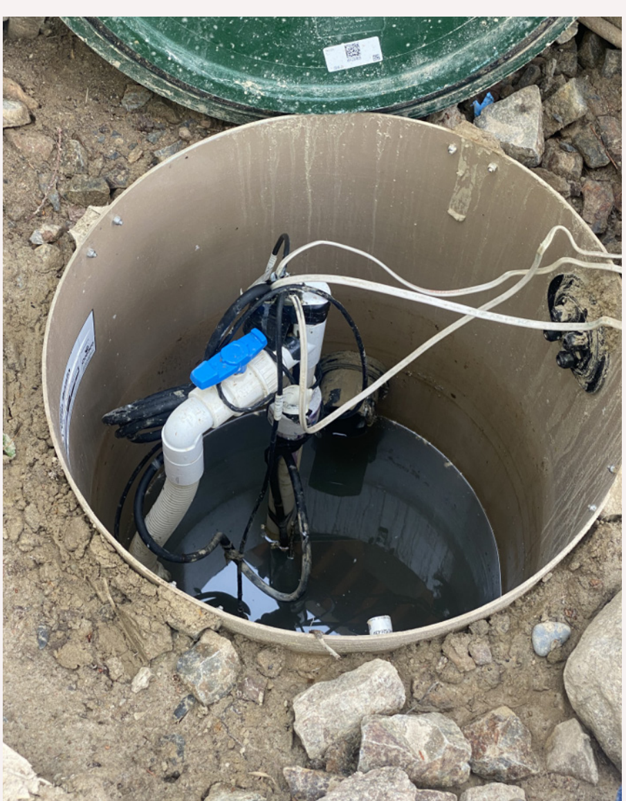
Individual Grinder Pump Station
