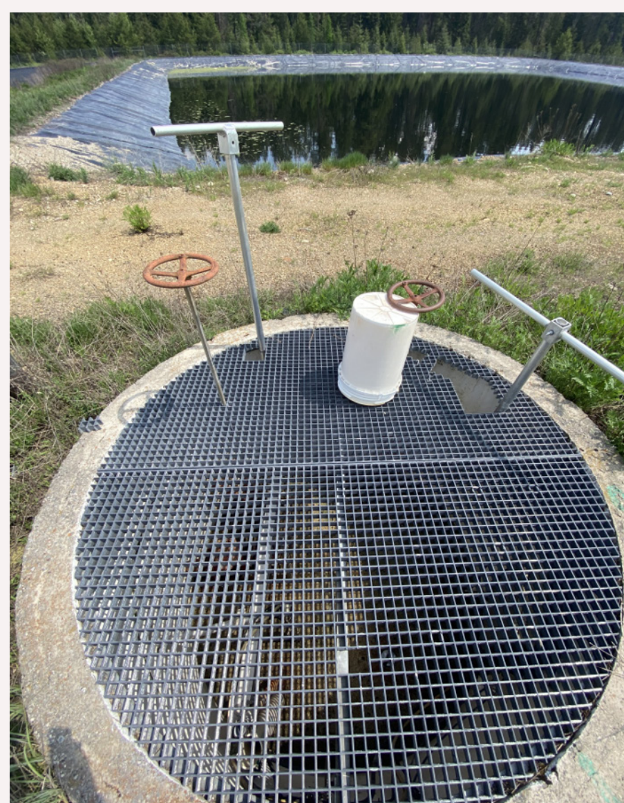
WWTP Valve Vault and Lagoon
