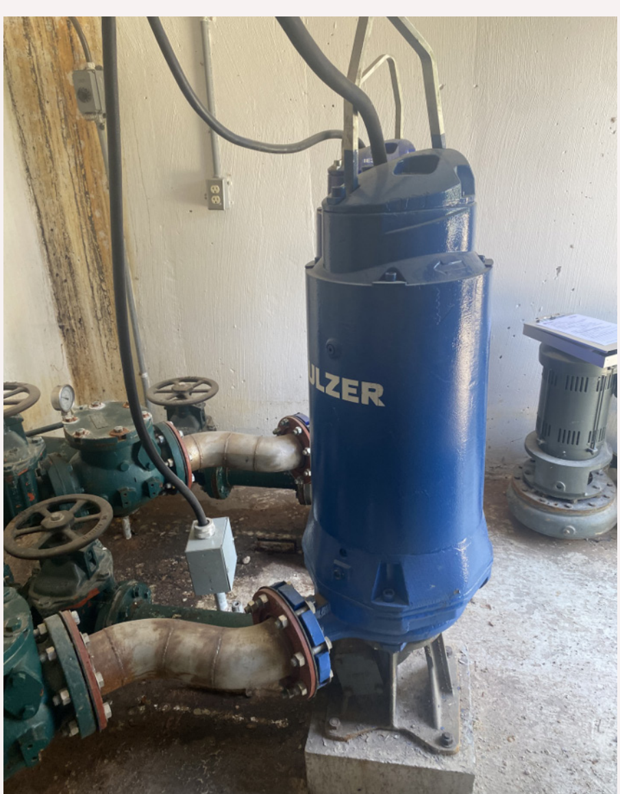
Lift Station Pump
